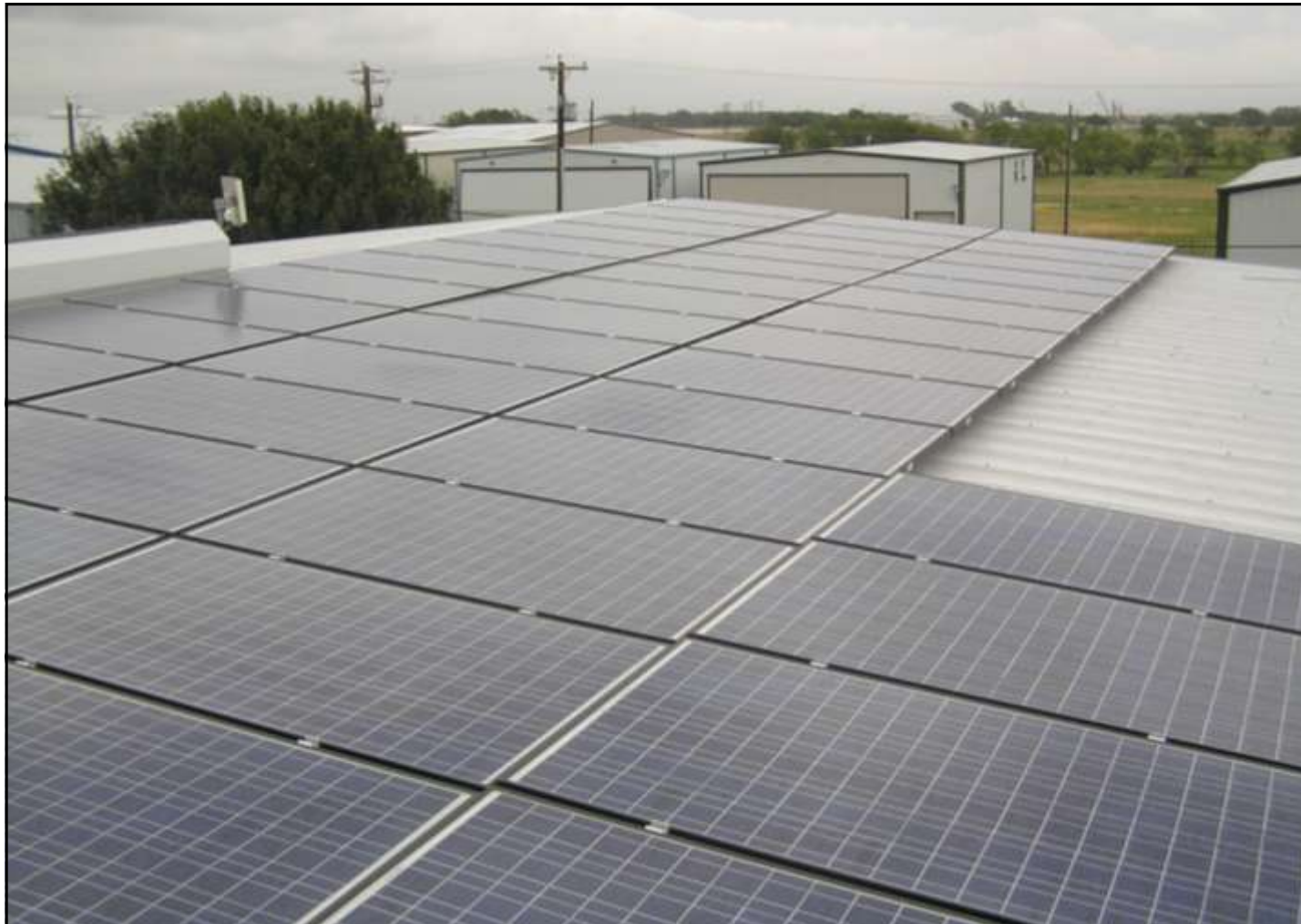
Solar panels cover a hangar roof as one HAPA member goes green. Page 4
