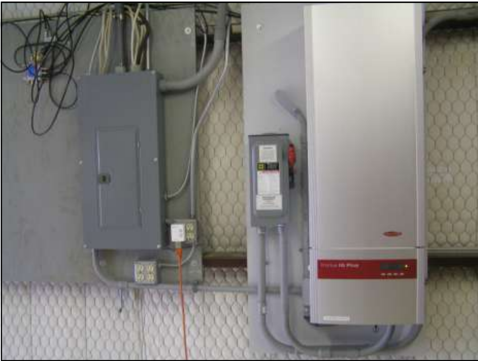
The inverter which converts incoming DC to AC with output reading.
