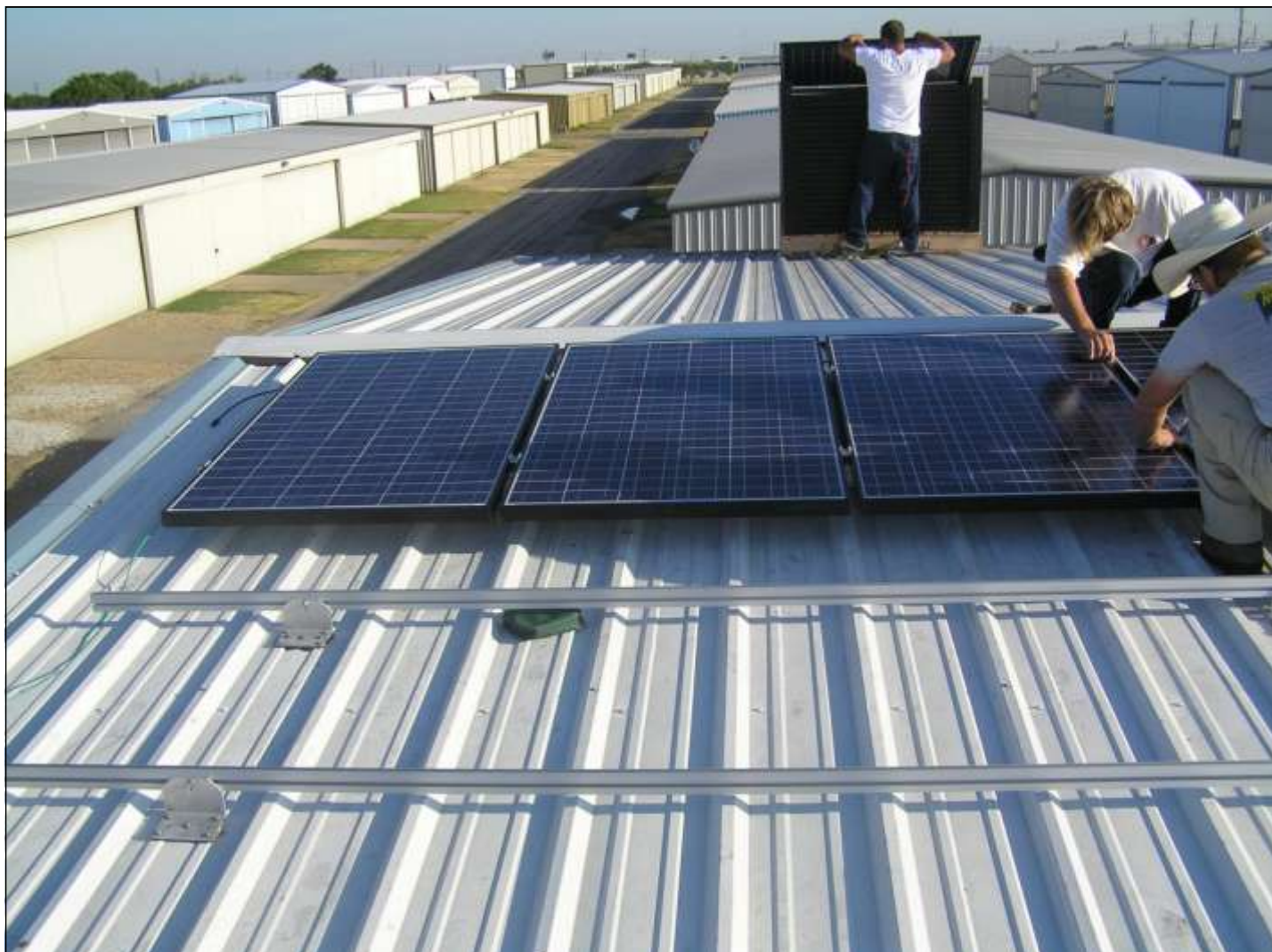
Workmen spent 3 days installing and wiring the three sets of 18 modules in series.
